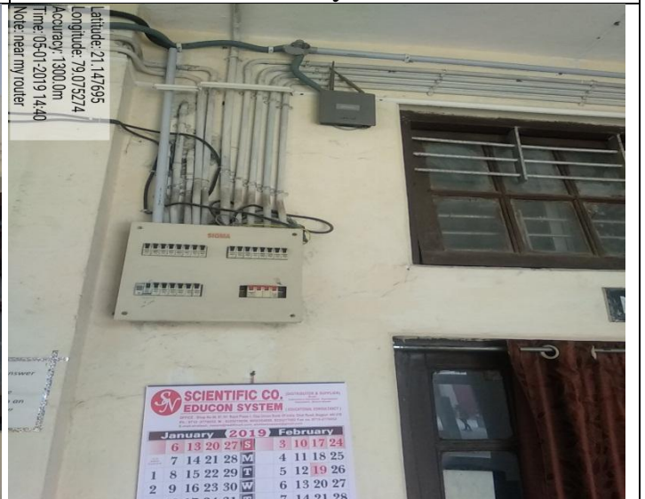
Router near NAAC Room
