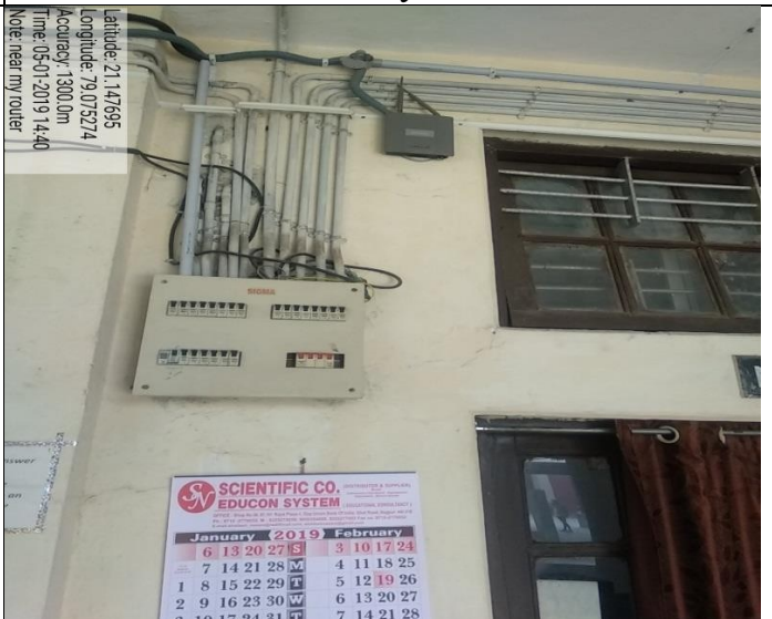
Router near NAAC Room
